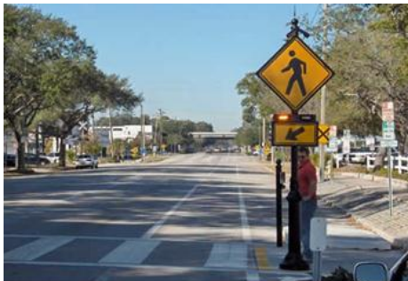
Rectangular Rapid Flashing Beacon
