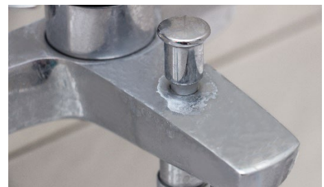
Mineral scale on water faucet
